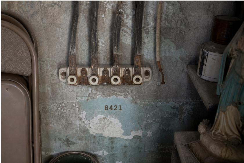
Figure 6 · Connection bar in the Caseta. The fifth transmission route has been resolved for the controlled separation test; under the color, 8421 is revealed.
